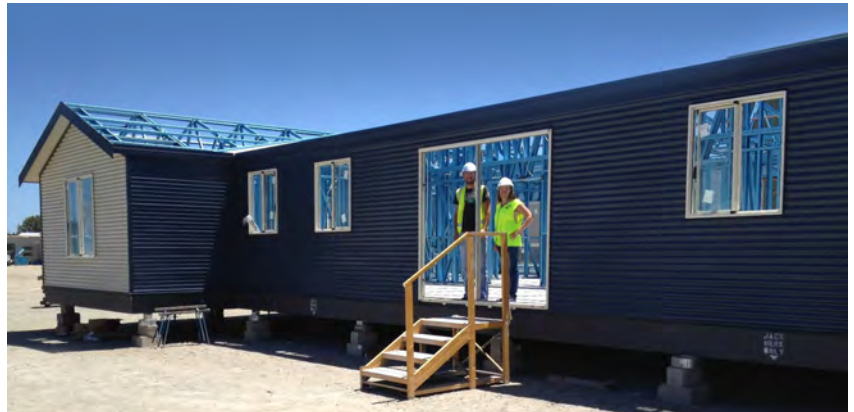
Photo: Tye Santos and Jenna Freind of Dowerin with their partially built home at TR Homes in Maddington. Photo supplied by TR Homes.
