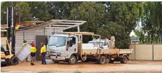
Above: Shire staff installing the new public toilets at jumping pillow and playground
