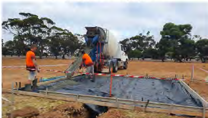
Above: Laying the pads for the BBQ and picnic areas for the playground.
