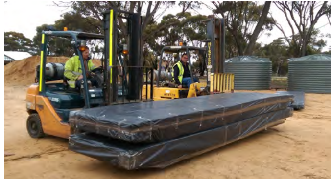
Rex Walker and Darren Spencer from Lake Grace Transport delivering building materials.
